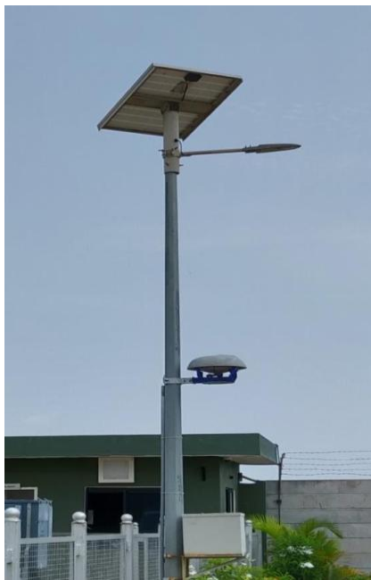
Figure 3: Installed Environmental Sensor
